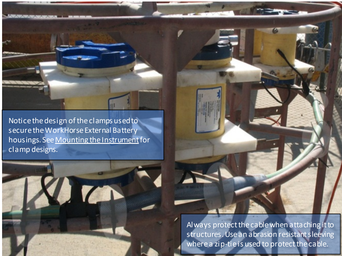
Figure 12. Cables Protected with Abrasion Resistant Sleeving
